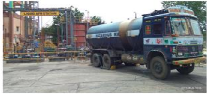
Mechanized system for unloading and feeding AFR weigh feeder and Rotary airlock. 5KL/Hour through calciner and 10KL/Hour through Kiln, Storage Capacity of 50KL Storage capacity of 100MT.
