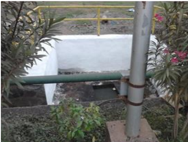
Drain Water Harvesting Pit
