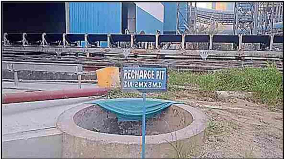
Rain Water Recharge Pit with connecting drain near stacker reclaimer
