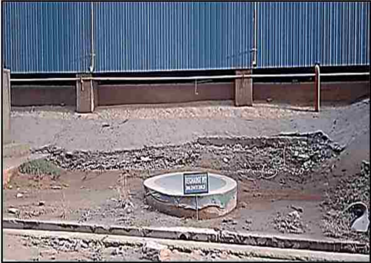
Rain Water Recharge Pit with connecting drain near stacker reclaimer
