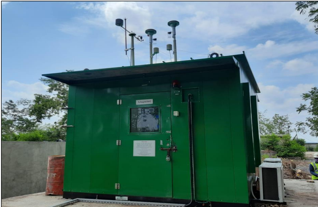
CAAQMS -01 installed at Plant Main Gate
