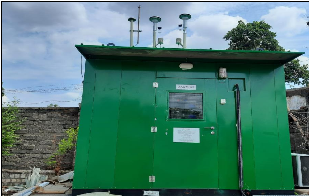
CAAQMS -02 installed at CPP Area
