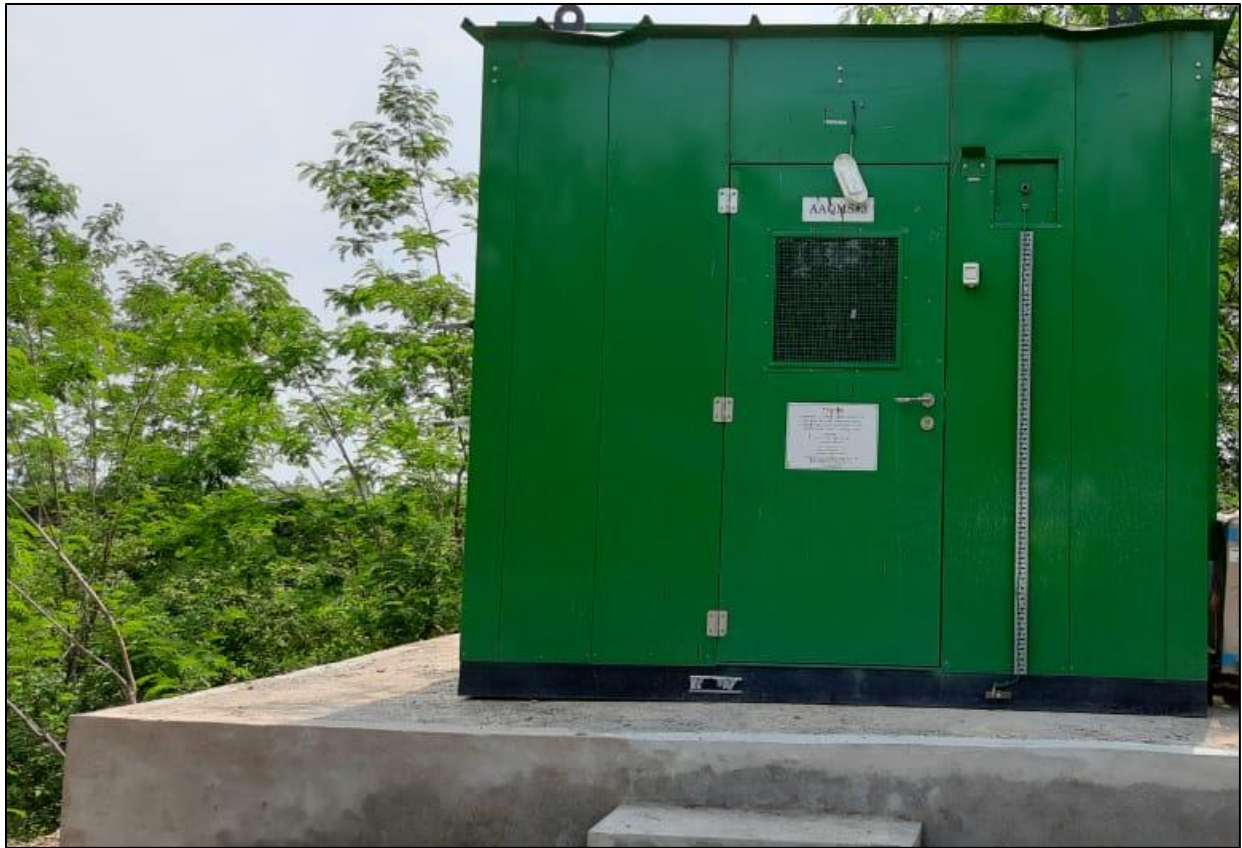
CAAQMS -03 Installed at Crusher Area (Mines)
