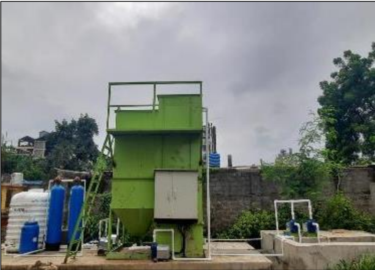
Sewage Treatment Plant Installed at Admin Building Main Gate
