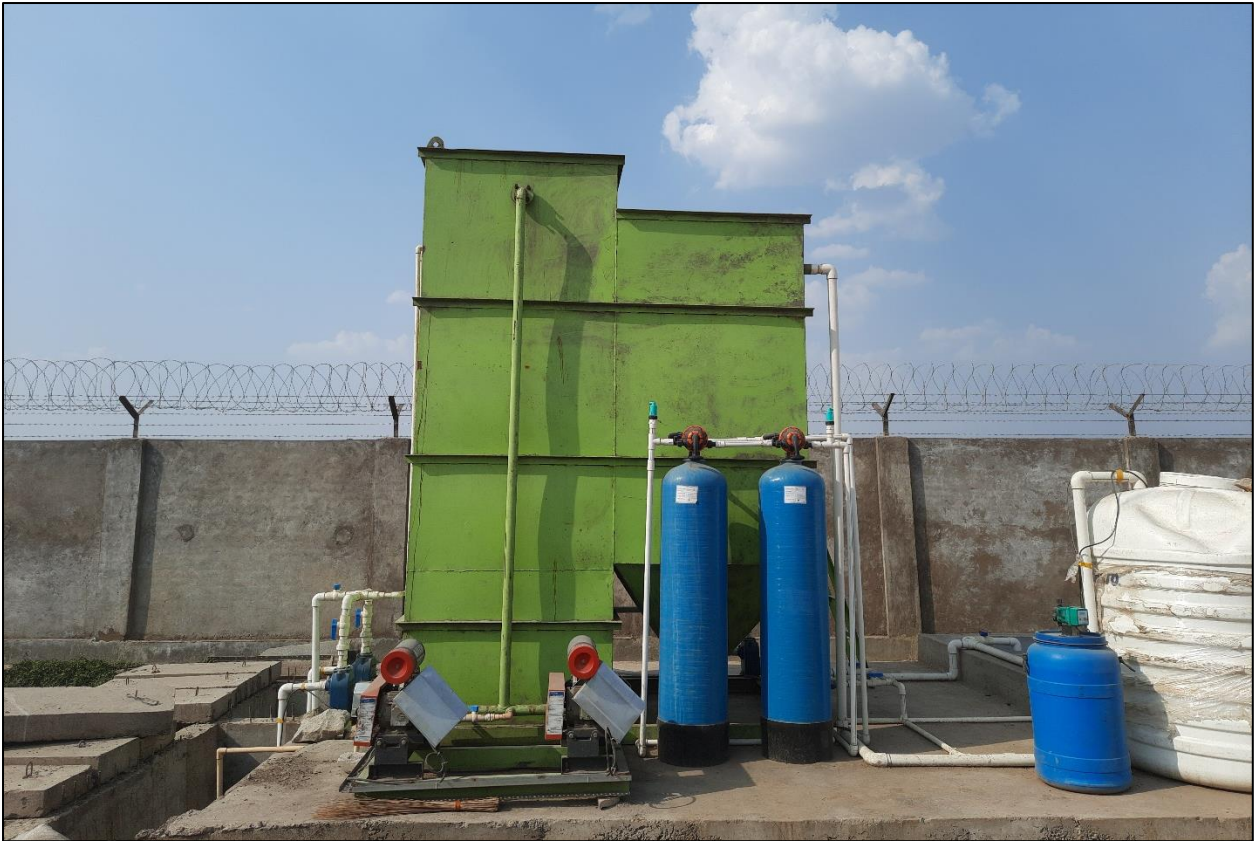
Sewage Treatment Plant Installed at Temporary Hutment Area
