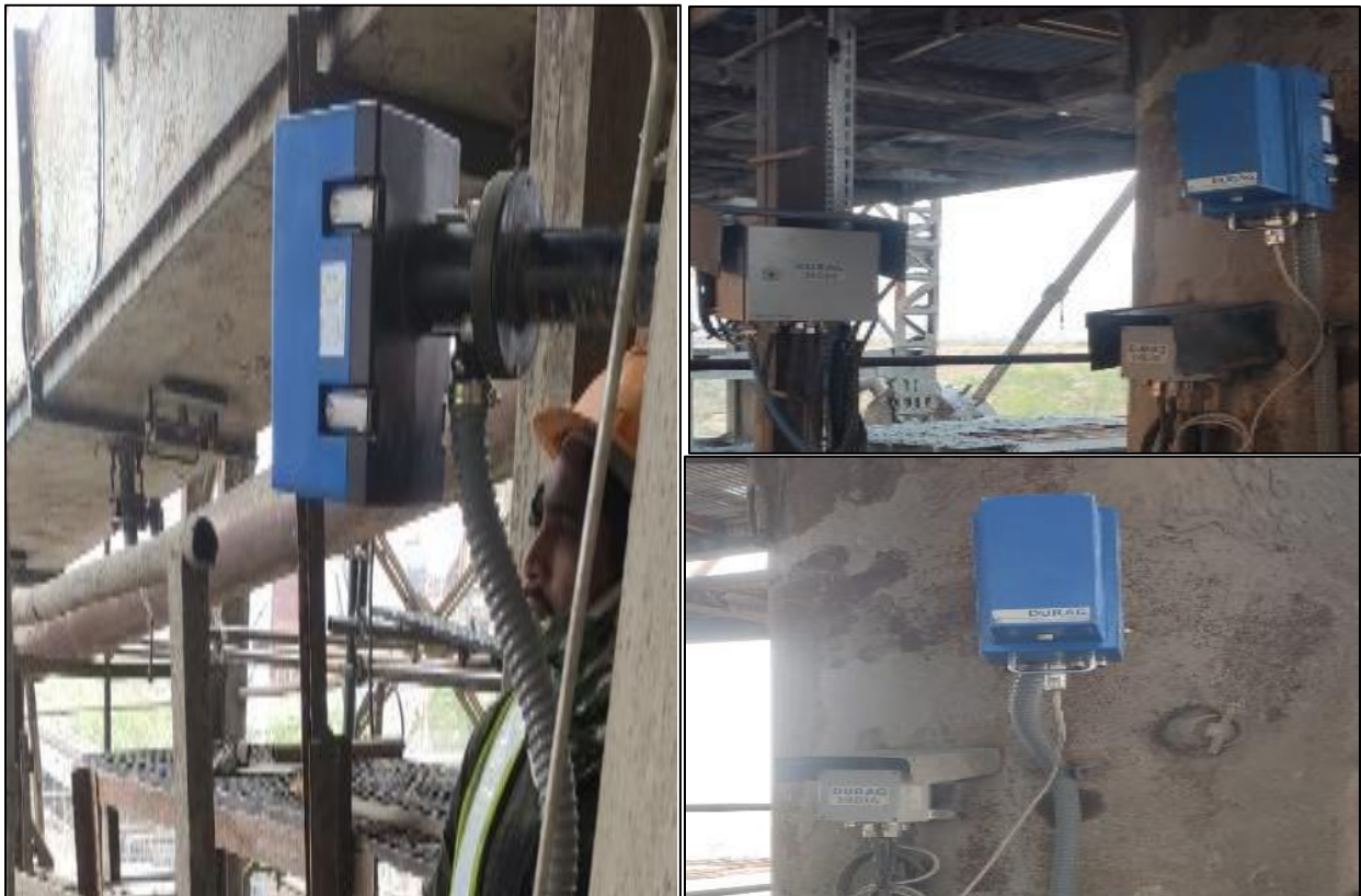
Installation of Opacity Meter for PM Monitoring at Major Stacks
