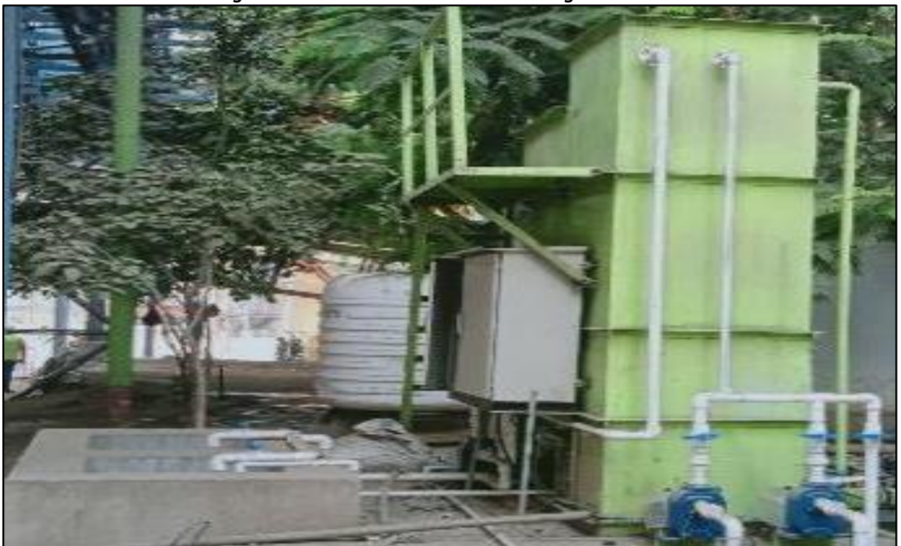
Sewage Treatment Plant Installed at CCR Area
